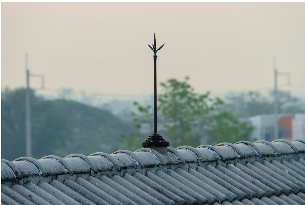
Figure 2. Image of a lightning rod set on a roof.
